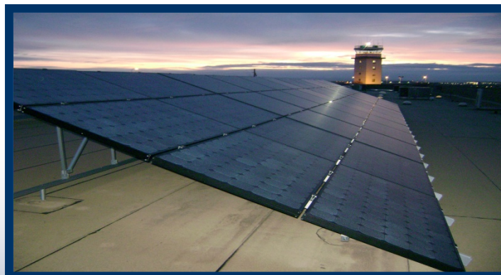
CDC Pools – 9.2 kW system
