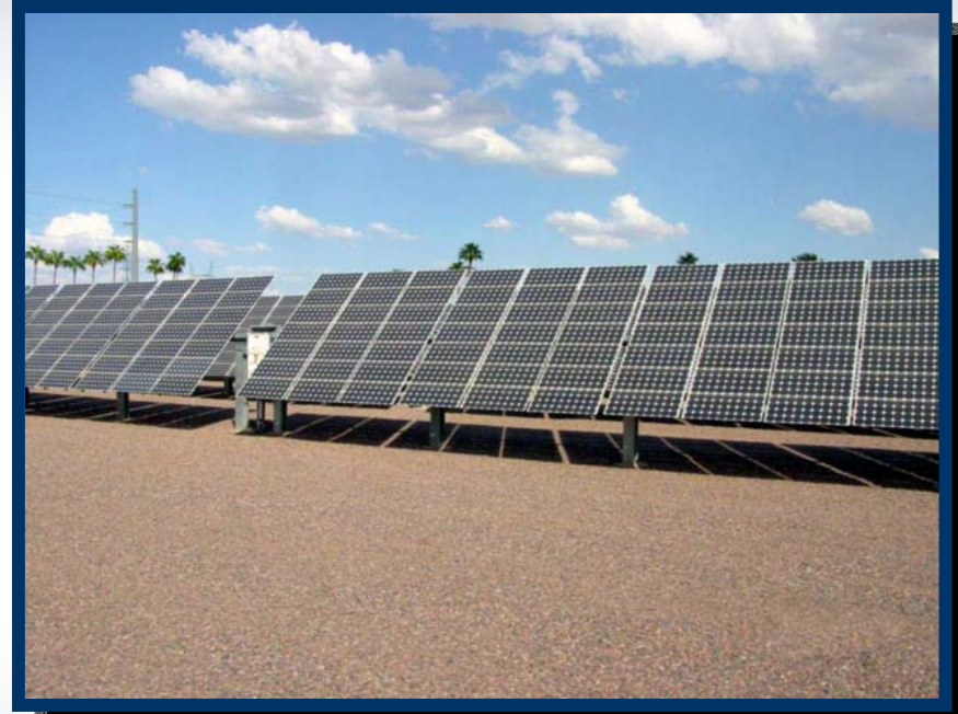
Rogers Substation, Mesa 400 kW
