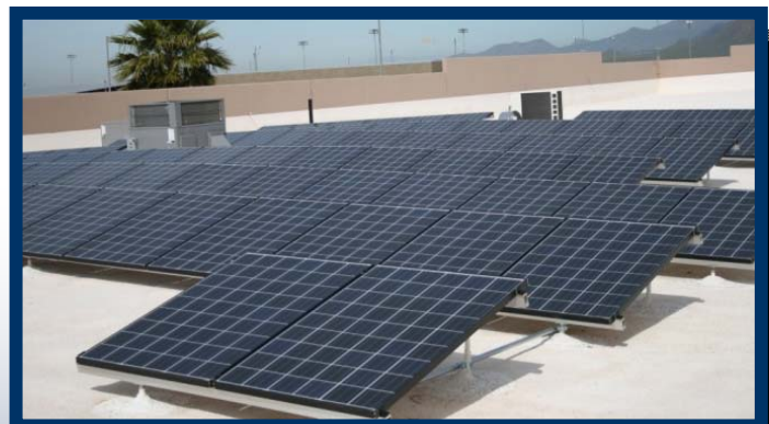
Integrity Building Corp. – 19 kW system
